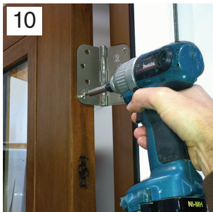
Step 10 Re-hang door on hinges. Double check that hardware fits and latches properly.
